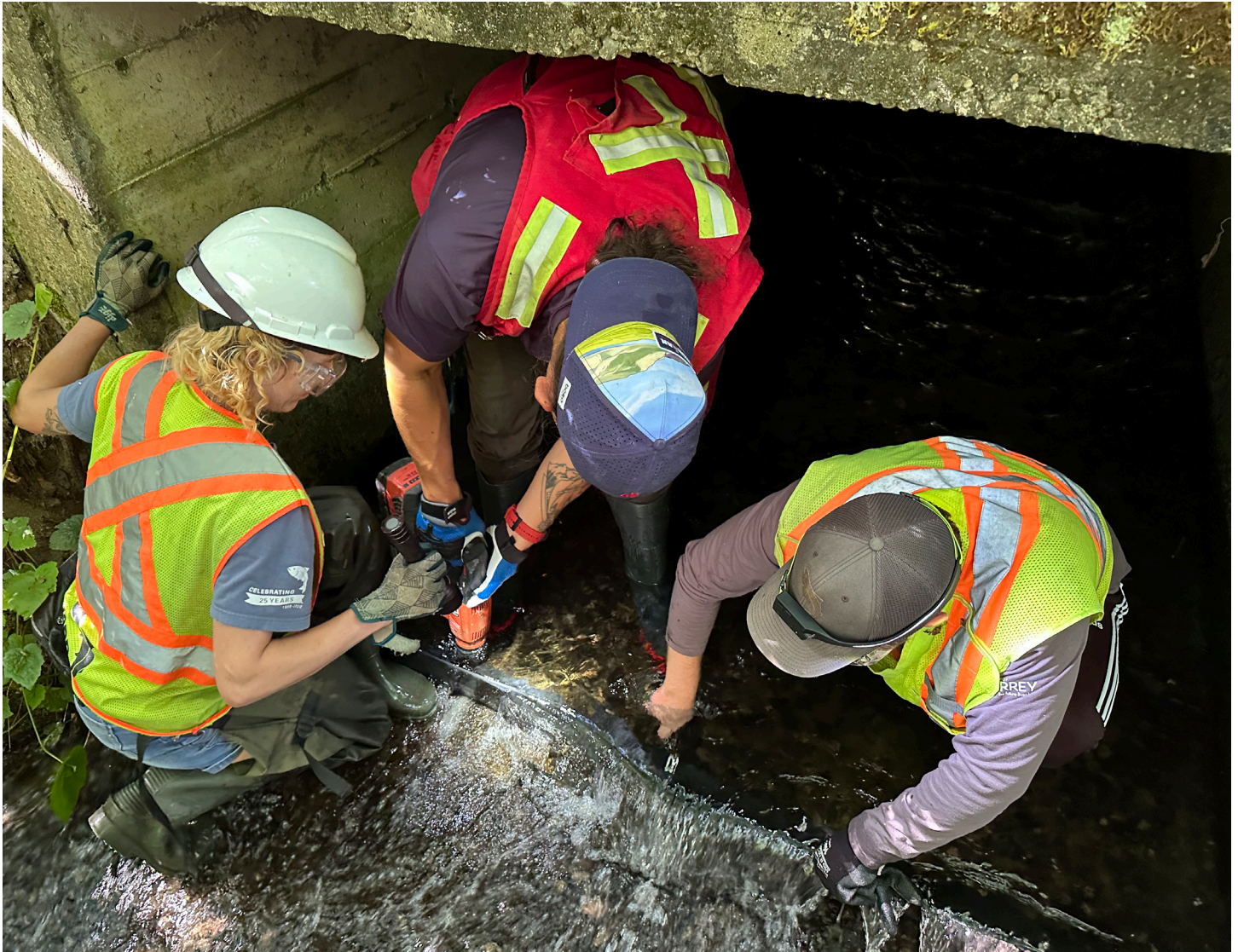
Students installing Flexi Baffles in Bon Accord Creek, Surrey, British Columbia, as part of the Salmon Habitat Restoration Program. The Flexi Baffle can be quickly installed using hand tools.
